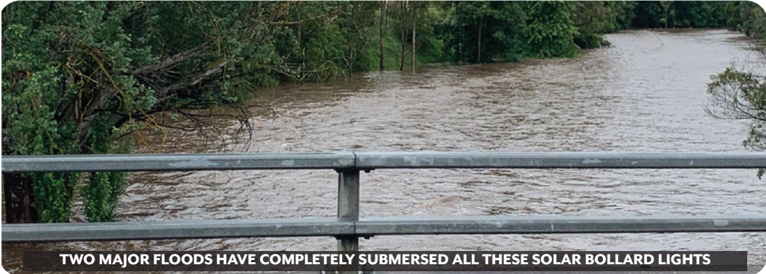
73 SBL2 SERIES SOLAR BOLLARD LIGHTS INSTALLED ALONG FLOOD PLAIN
