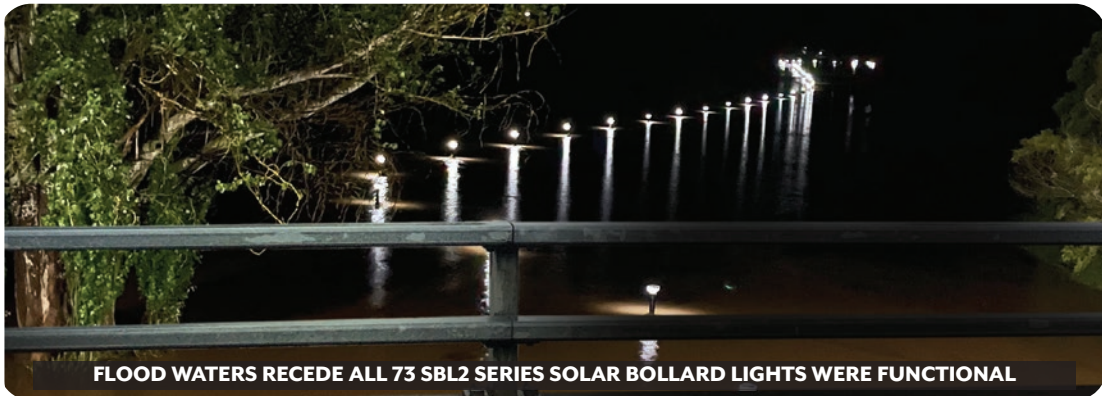
TWO MAJOR FLOODS HAVE COMPLETELY SUBMERSED ALL THESE SOLAR BOLLARD LIGHTS
